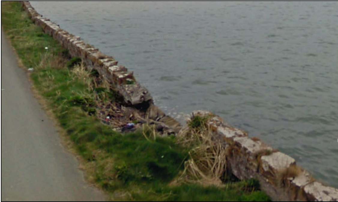
Figure 1.13: Damaged section of the existing seawall along the Channel road (© Google Earth)
