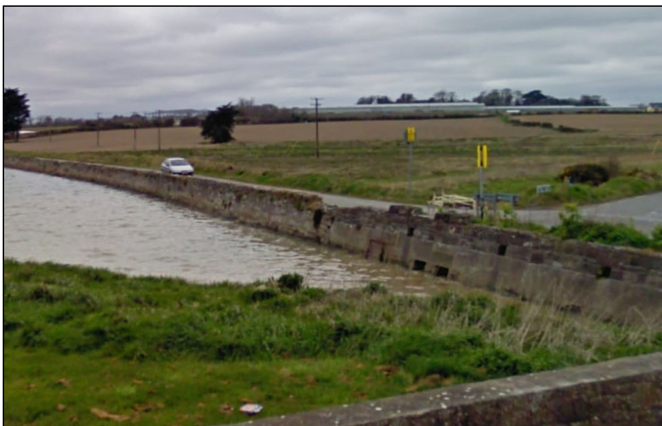
Figure 1.12: The existing seawall at the junction of Spout lane and Channel road (© Google Earth)
