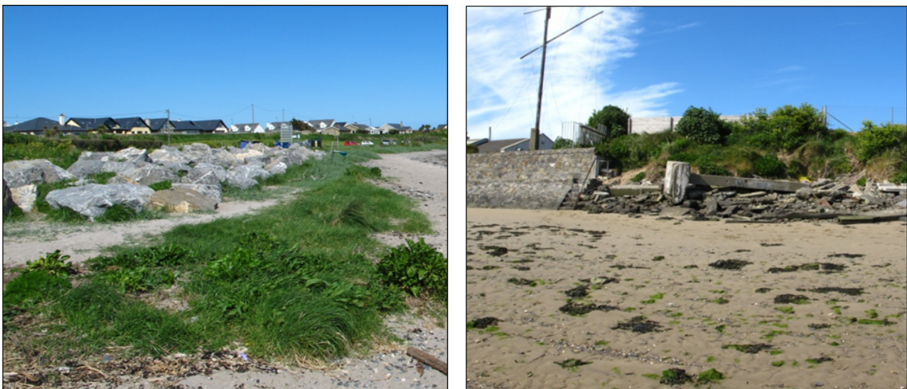
Figure 1.9: Existing coastal defences at the car park and boat club at Rush south
